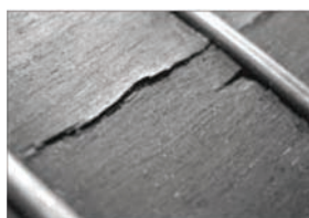
Frett Board cracks
